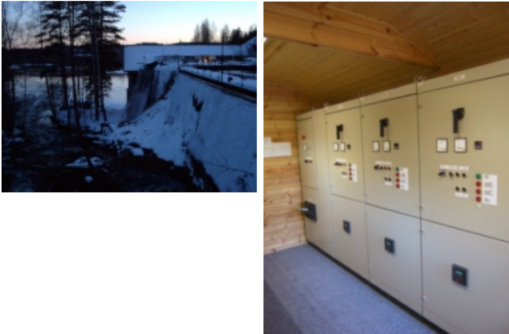
Figure 1.7. A small-scale hydropower plant offers the possibility to apply for the power line communications system under research and development. Picture of a small-scale hydropower plant in a rural area (left). The mains switching board of the plant (right).
