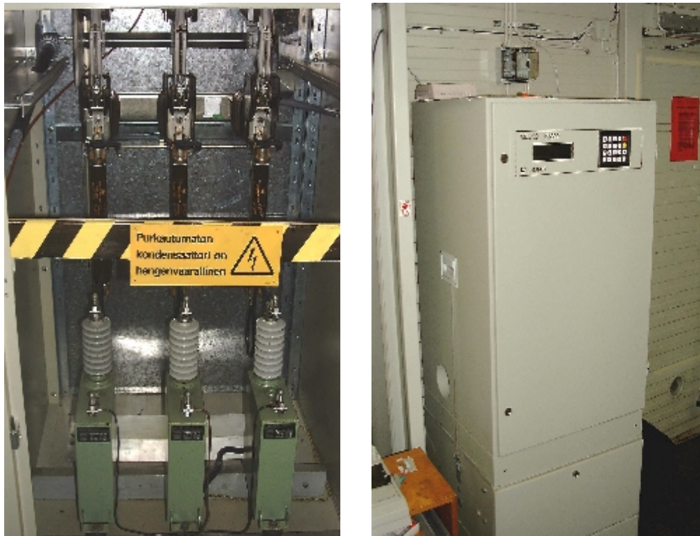
Figure 1.1. Coupling unit (left) and substation (right) of Melko™ load management system. The Melko™ systems are commonly used in Finnish distribution companies.
